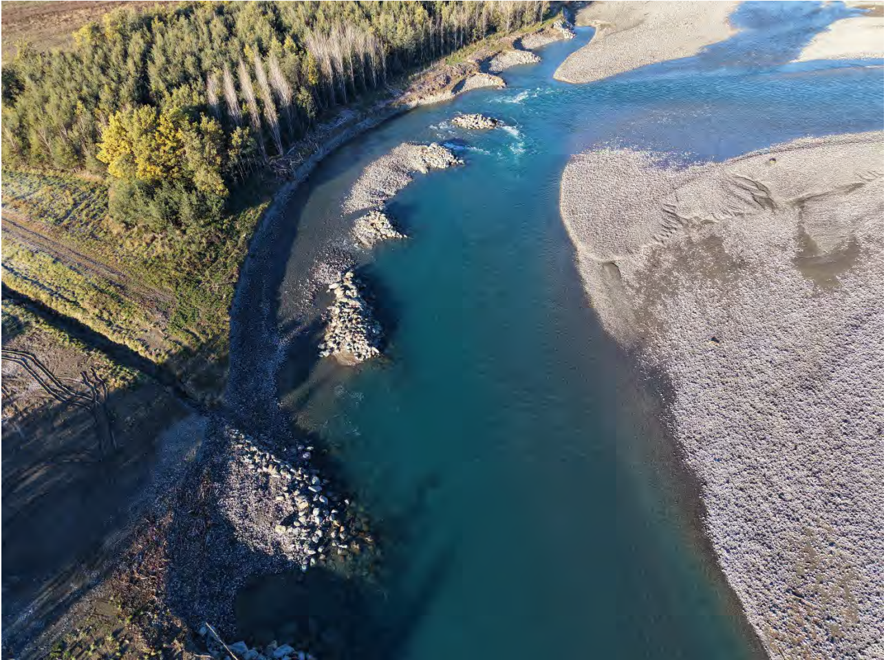
Figure 12: Wairau River TRB below Waihopai Confluence, significant loss of crucial berm area near Groyne 23 & 24 (June 2026)
