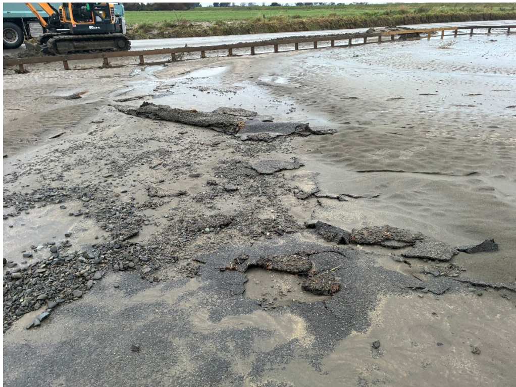
Damage to the seal of the carpark due to floodwater
