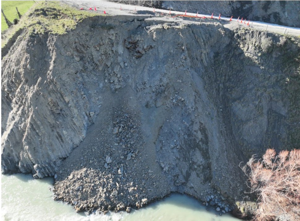
Figure 2- Recent dropout Awatere Valley Road
