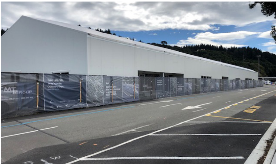
The new temporary terminal is scheduled to open in early May with just the interior fit out to complete
