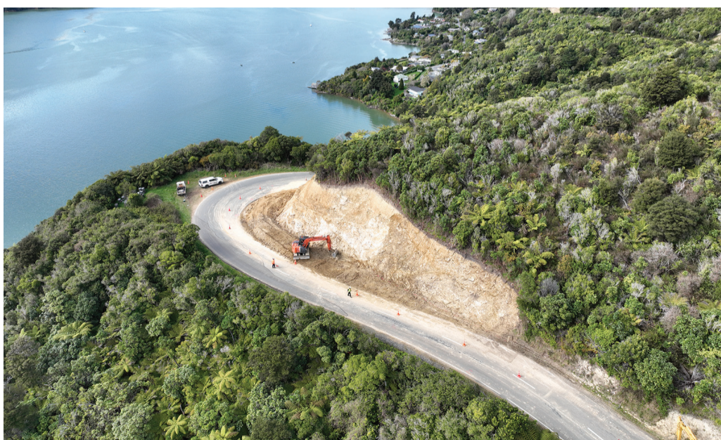
Repairs to Marlborough Sounds roads are a key part of Council's Long Term Plan 2024/2034
