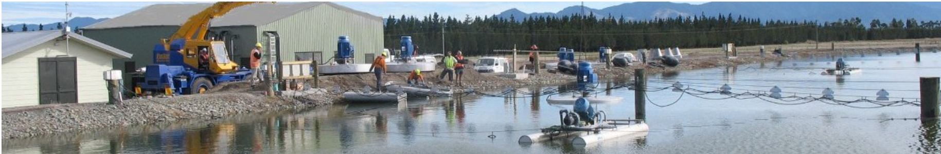
Photo: Sewerage Ponds, Hardings Road, Blenheim
