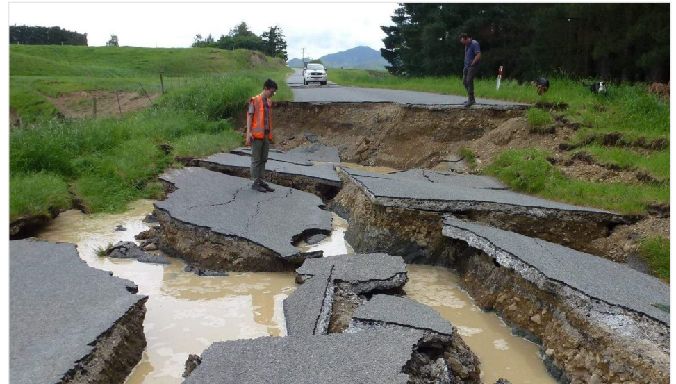
A road damaged in the 2016 Kaikōura earthquake. Source: Tonkin + Taylor - Copyright: Tonkin + Taylor 2017
