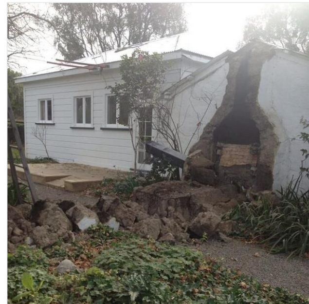
A badly damaged house in Seddon following the 2013 earthquake. Source: pic.twitter.com/PpQzONVaVs
