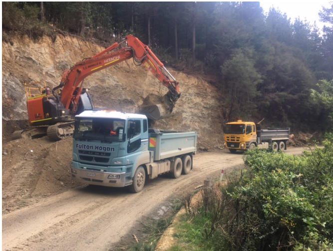
Slip clearance on Kenepuru Road just before Mahau Road (RP 12.8)
