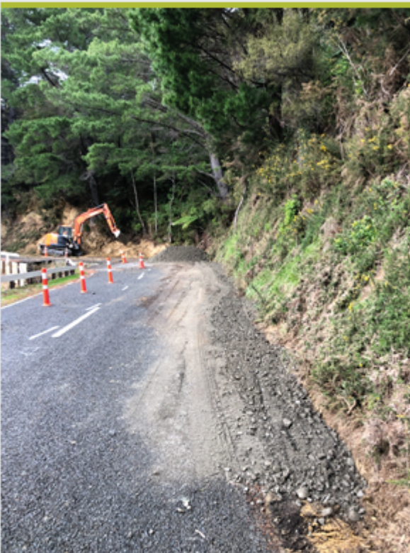
At the 12.8km mark from the Linkwater end of Kenepuru Road, the road width has been reinstated by taking the bank back by about 2m and numerous trees have been removed
