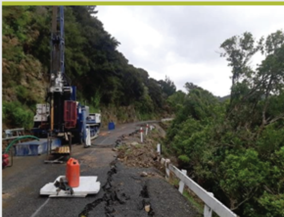
Drill rig working on site at the Water Tank slip 20.5km from Linkwater
