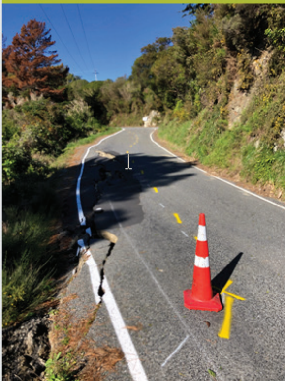
Before: Mistletoe Bay under slip
