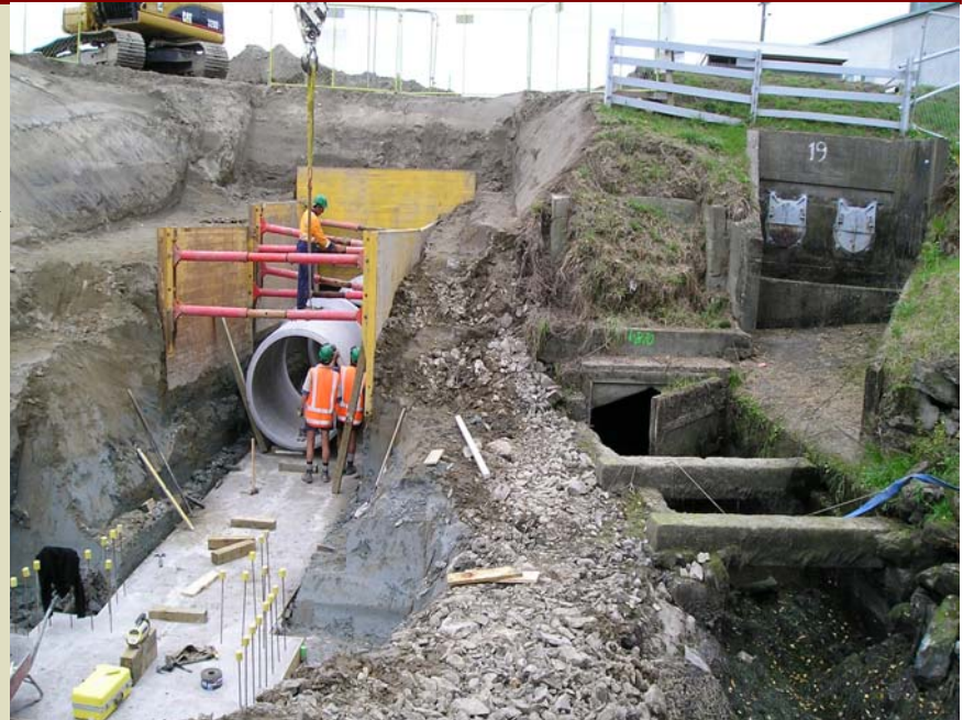
Contractor, Fulton Hogan installs a 1600mm diameter pipeline on a reinforced foundation bed, doubling the capacity of the Grovetown Lagoon's southern outlet. On top of the pipe, adjusting the width of shields which held the walls of the six metre deep trench in place, is excavator operator Peter Strange. Below are job foreman John Moses and carpenter, Trevor Woodhouse.
