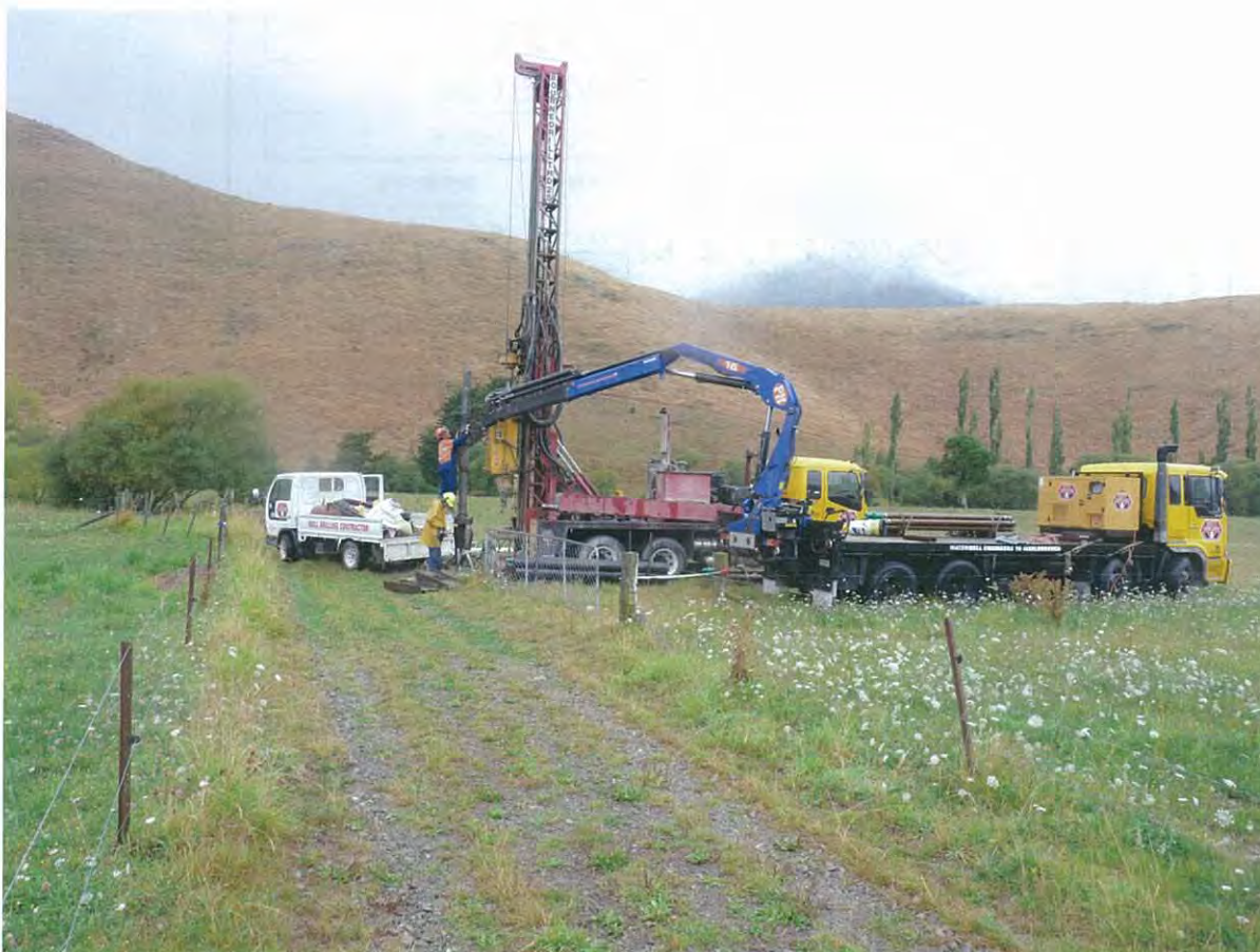
Figure 7 : Fitting Screen In Second Test Well (O27w/0119) February 2012
