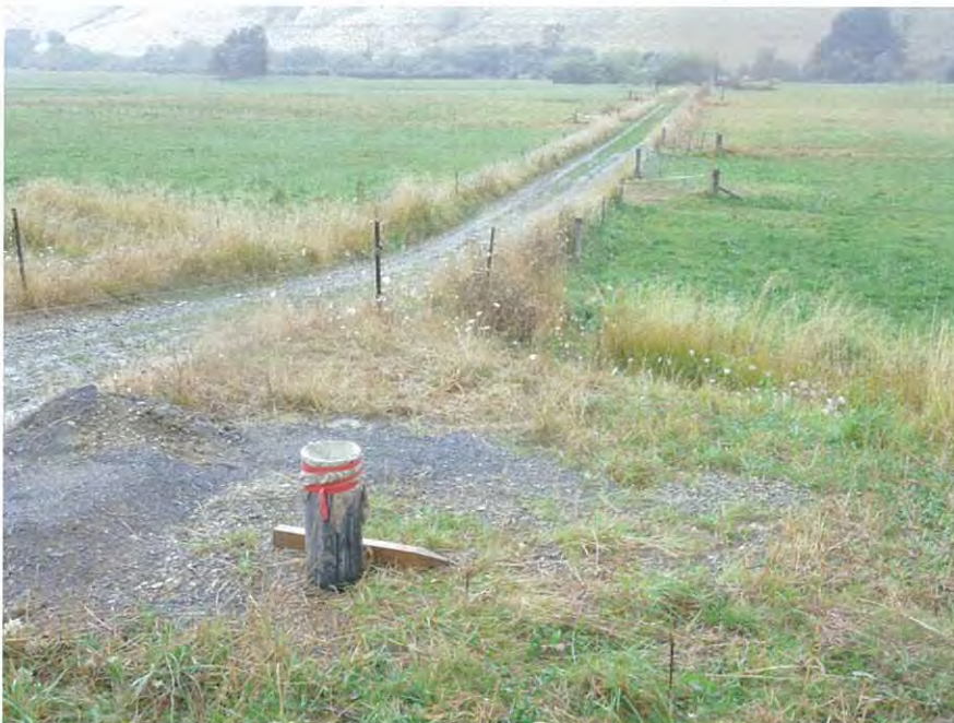
Figure 5 : Well 10323 With Rai River & Second Test Well Under Construction In Background (February 2012)
