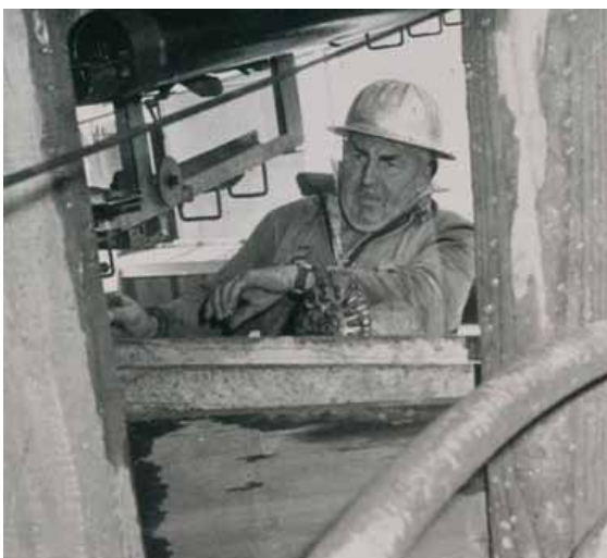
Figure 3.20 Mr G.R. Simpson drilling the new Blenheim library lift well (Courtesy of The Marlborough Express)
