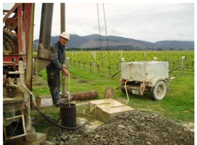
Figure 3.21: Colin Simpson drilling one of three new MDC Renwick domestic supply wells in 2008
