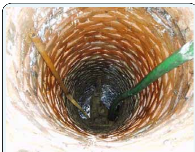
Figure 3.3: Brick lined Benmorven well (June 2010). Photograph taken as well was being pumped to verify its depth. The green hose is the pump intake and the static level is marked by the darker shade of orange sitting just below the top of the metal pipe.
