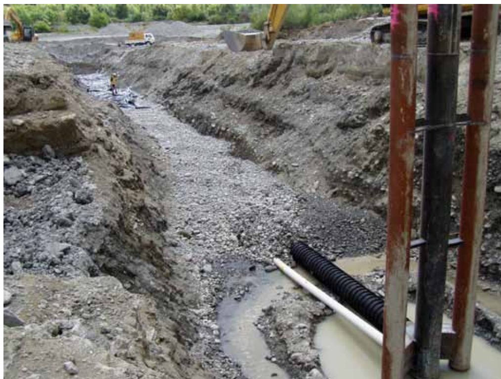
Figure 3.12: Awatere River infiltration gallery under construction. Note size of person standing in the trench.
