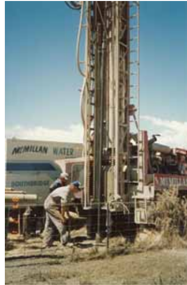
Figure 3.29: McMillan Water Wells Ltd mud/air rotary rig drilling piezometers for the MCRWB.
