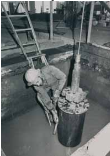
Figure 4.1: Mr C.G. Simpson working on the Blenheim Library lift well (The Marlborough Express)
