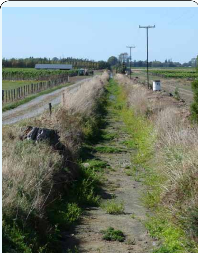
Figure 25.7: Fairhall Co-op Drain looking downstream towards Battys Road. The channel is dry until opposite the white drum on the right hand bank, where water is ponding. Actual channel flow doesn't occur until the 3rd power pole in the distance where light can be seen reflecting off the water surface.
