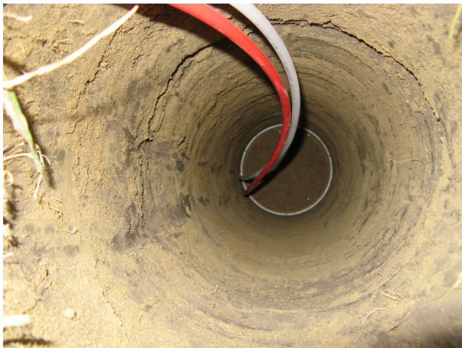
Figure 7: This photograph is looking down into the hole where a drainage flux meter (DFM) is being installed. The top of the convergence ring is at a depth of 1.0 m. Soil from this hole was originally collected at 10 cm depth increments. These samples were placed into plastic buckets, and then repacked into the hole, in the same order and at a similar density to the original soil profile. Despite careful packing, some setting down period (perhaps the first winter) is expected.
