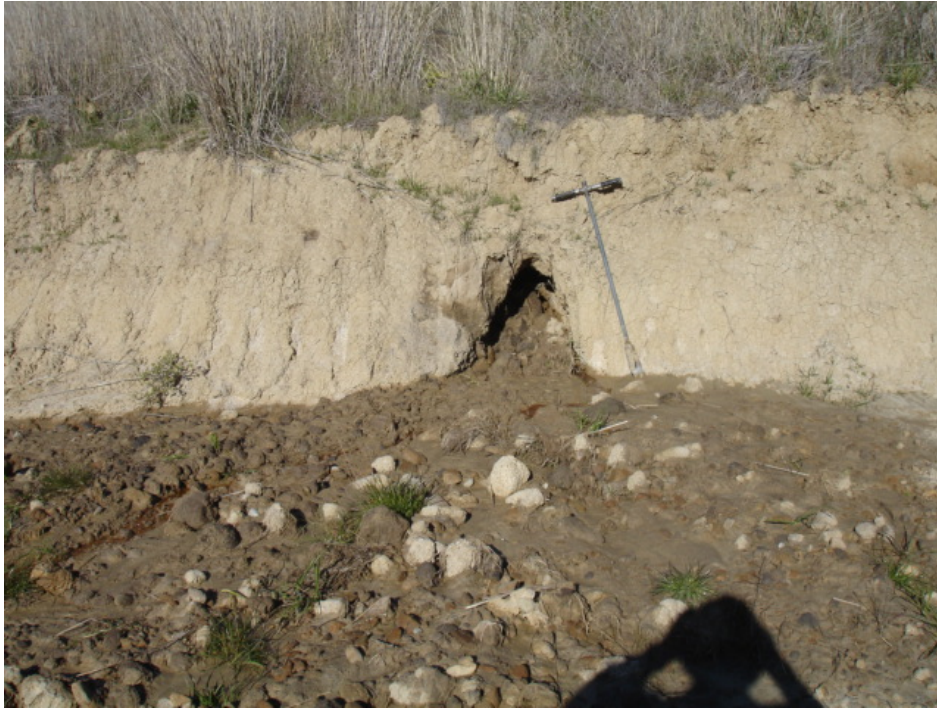
Figure 38. A piping channel on a lower slope with outflow water-transported debris (colluvium) deposited during heavy winter rains.
