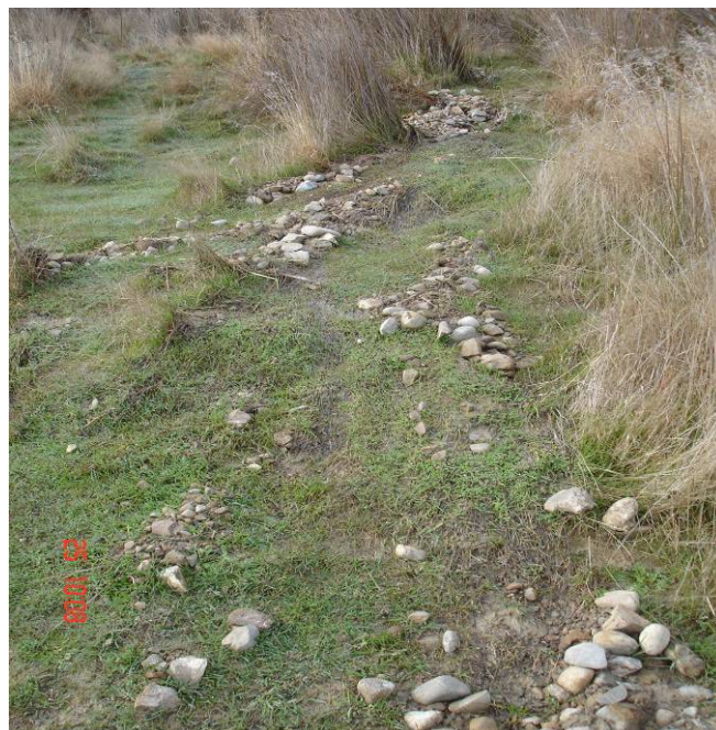
Figure 39. Recently deposited coarse material (colluvium) deposited mid slope, and transported by water from a small up-slope outlet pipe.
