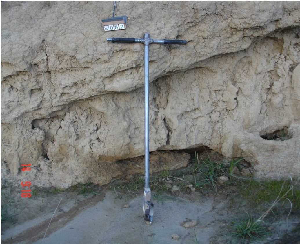
Figure 40. Silt deposited at a piping outlet as a result of soil dispersion. The fragic horizon has multiple layers.
