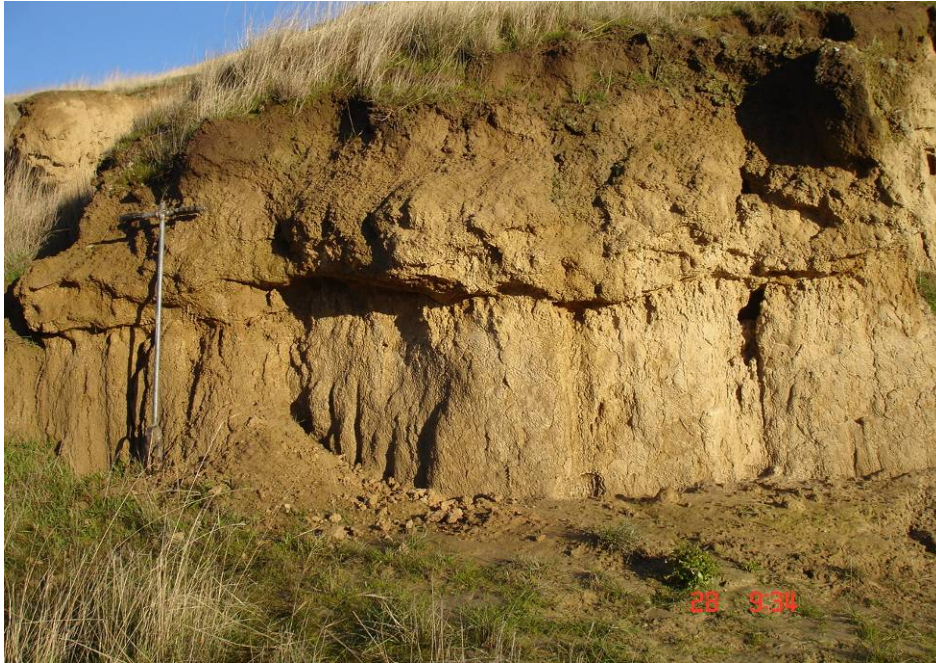
Figure 36. At this site, water in the saturated soil was flowing down-slope on the top of the pan and trickling down the face of the section, causing dispersion of the clay loam material beneath and undercutting the pan. The dispersed soil is being deposited as structureless caked material at the front of the section as headward erosion continues.
