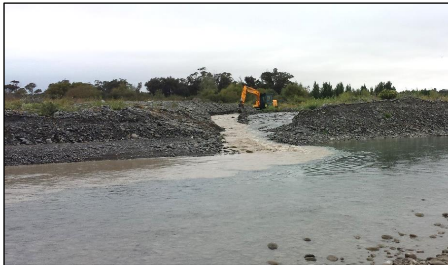
Figure 7. Maintenance works on an infiltration gallery, using an excavator to rip the bed, in a diversion channel adjacent to the lower Awatere River on 18 January 2016. A sediment plume can be seen entering the mainstem of the Awatere River in the foreground.
