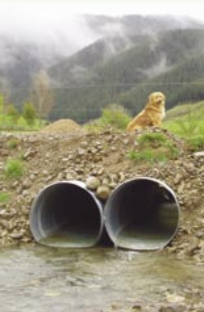
Culverts need to be installed correctly to allow fish passage
