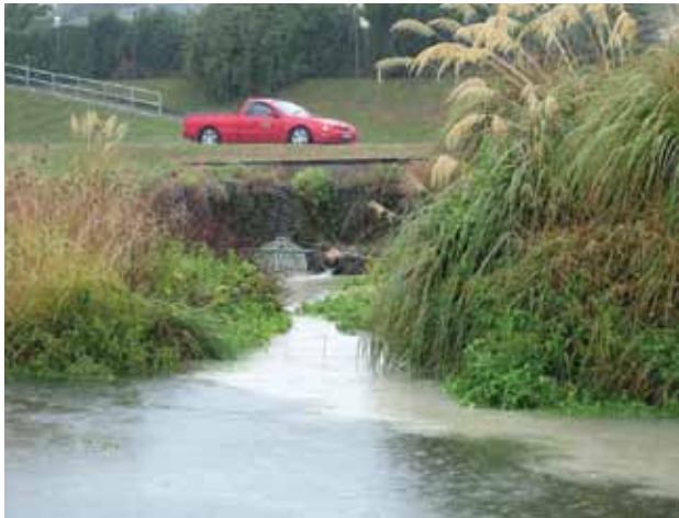
Stormwater discharge to the Taylor River
