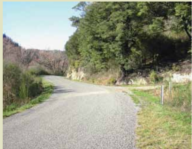
Onamalutu Road with a dwelling vehicle access (on right) in close proximity to a blind corner
