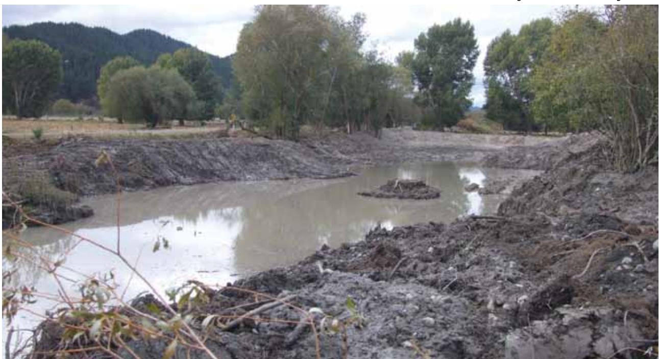
Illegal excavation of existing wetland
