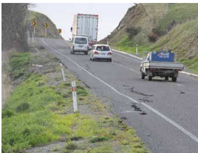
Earthquake damage SH1
