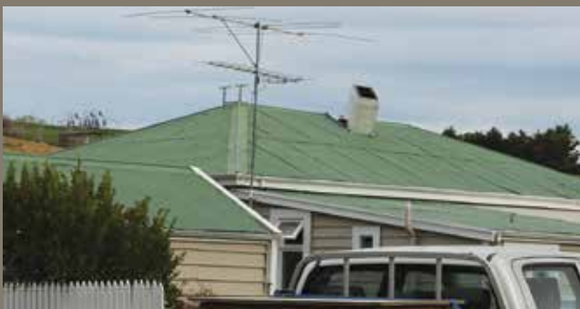
Toppled chimney as a result of the Seddon earthquake
