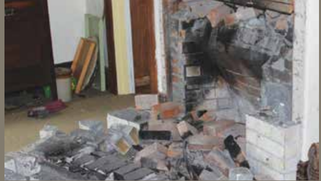
Damage from Grassmere earthquake
