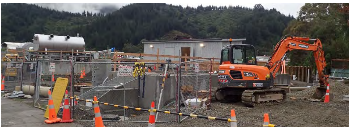
Figure 14: Upgrade of the sewerage network near the Waitohi River which flows into Picton Harbour.
