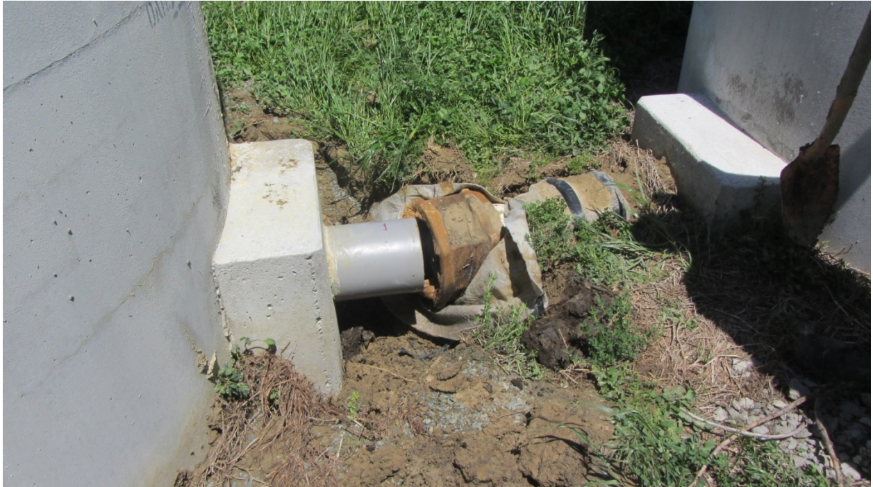
Figure 4-6 The effect of differential movement between the tanks and buried pipework
