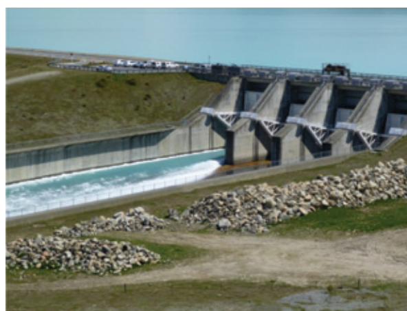
Figure 6.12: Crest Mounted Radial Gates – Pukaki Dam (provided by Meridian Energy)
