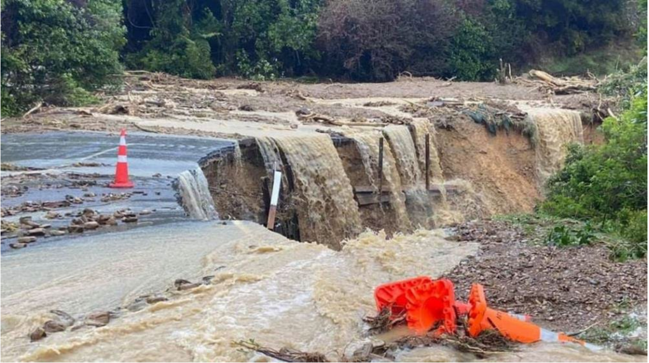
Figure 4-8: Section of Queen Charlotte Drive flooded with water and debris (2021)
