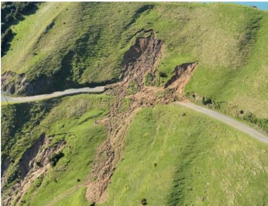
Figure 4-2: Natural Slope Instability on French Pass Road (2022)
