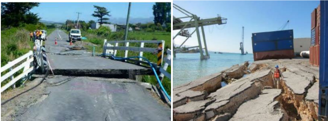
Figure 4-7: Liquefaction and Lateral Spreading implications to a bridge and a marine hub facility (Source unknown)
