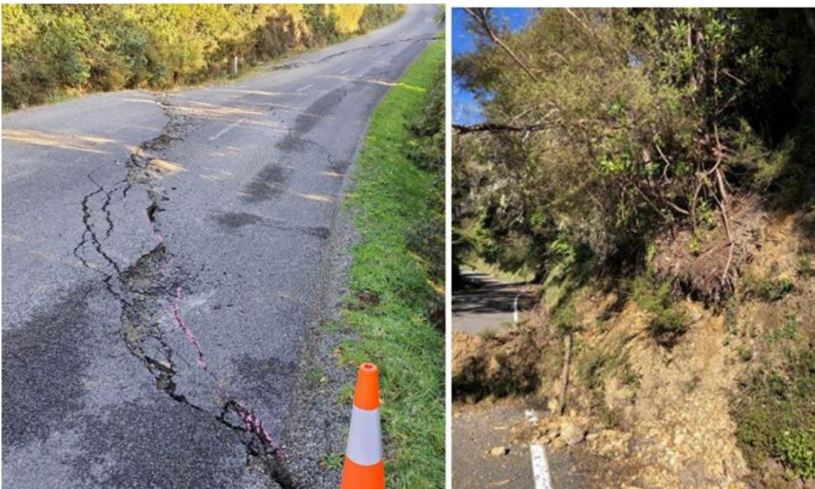
Figure 4-4: Human Induced Slope Instability (underslip and overslip on Kenepuru Road, 2022).
