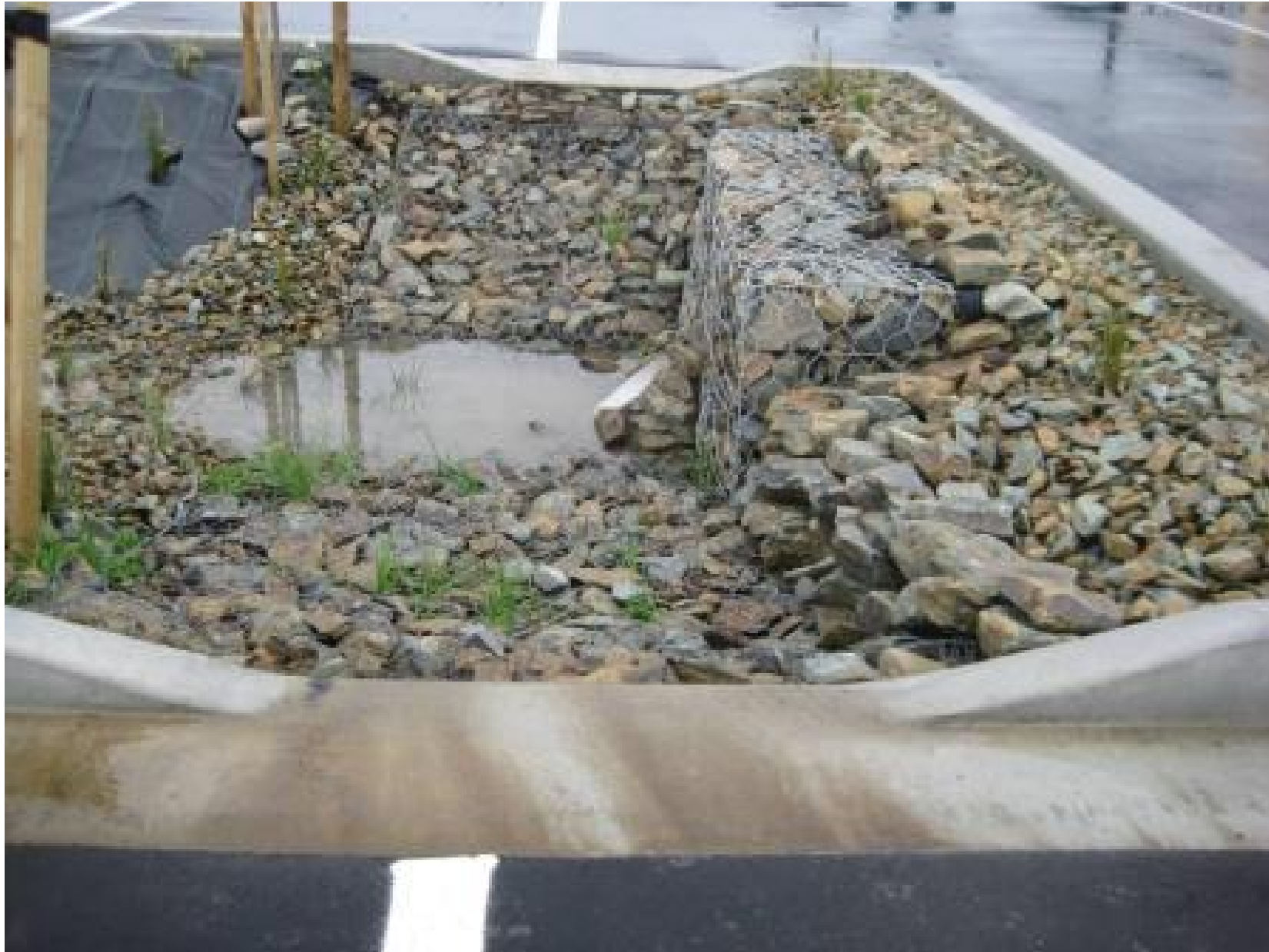
Storage Area – Stormwater Ponding – 9 August 2012
