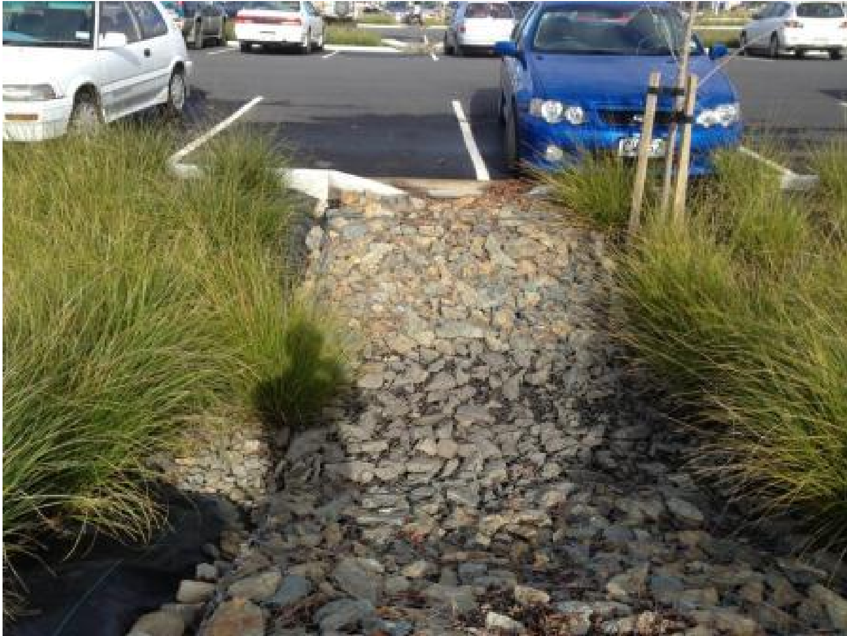
First Flush – Sediment Capture – Off Car Parks – 18 June 2013
