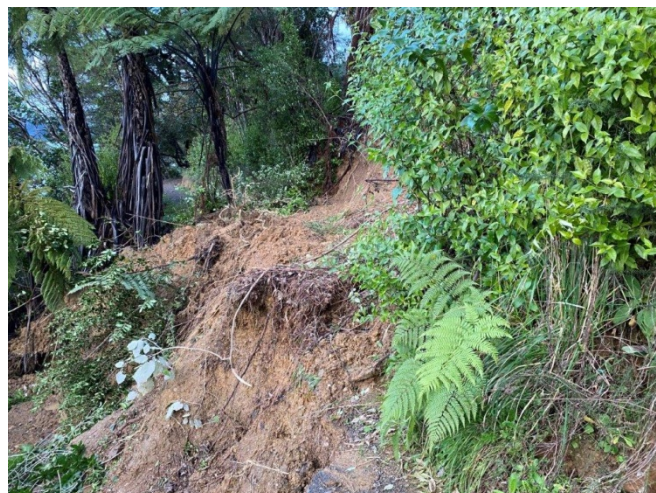
Link Pathway, Grove to Momorangi – Slumping
