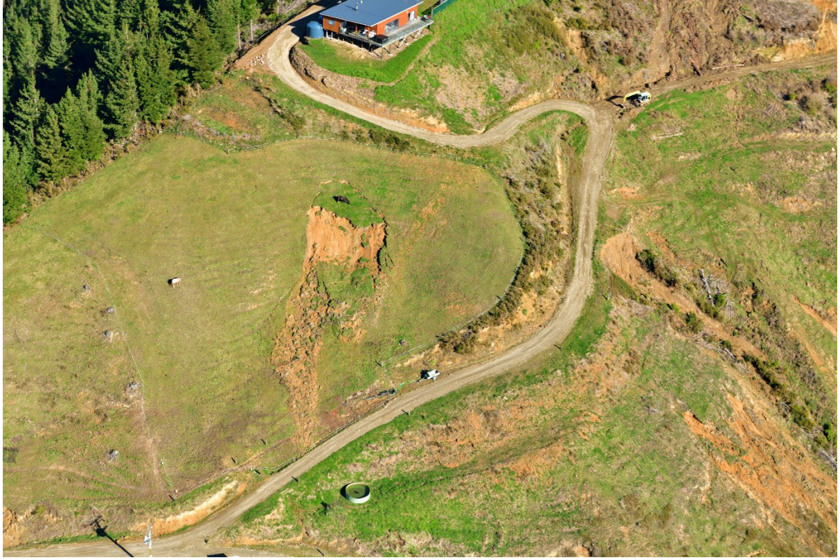
Figure A1.12 Deeper-seated landslide and incipient landslide/slump in pasture, also showing cracking, near Havelock.
