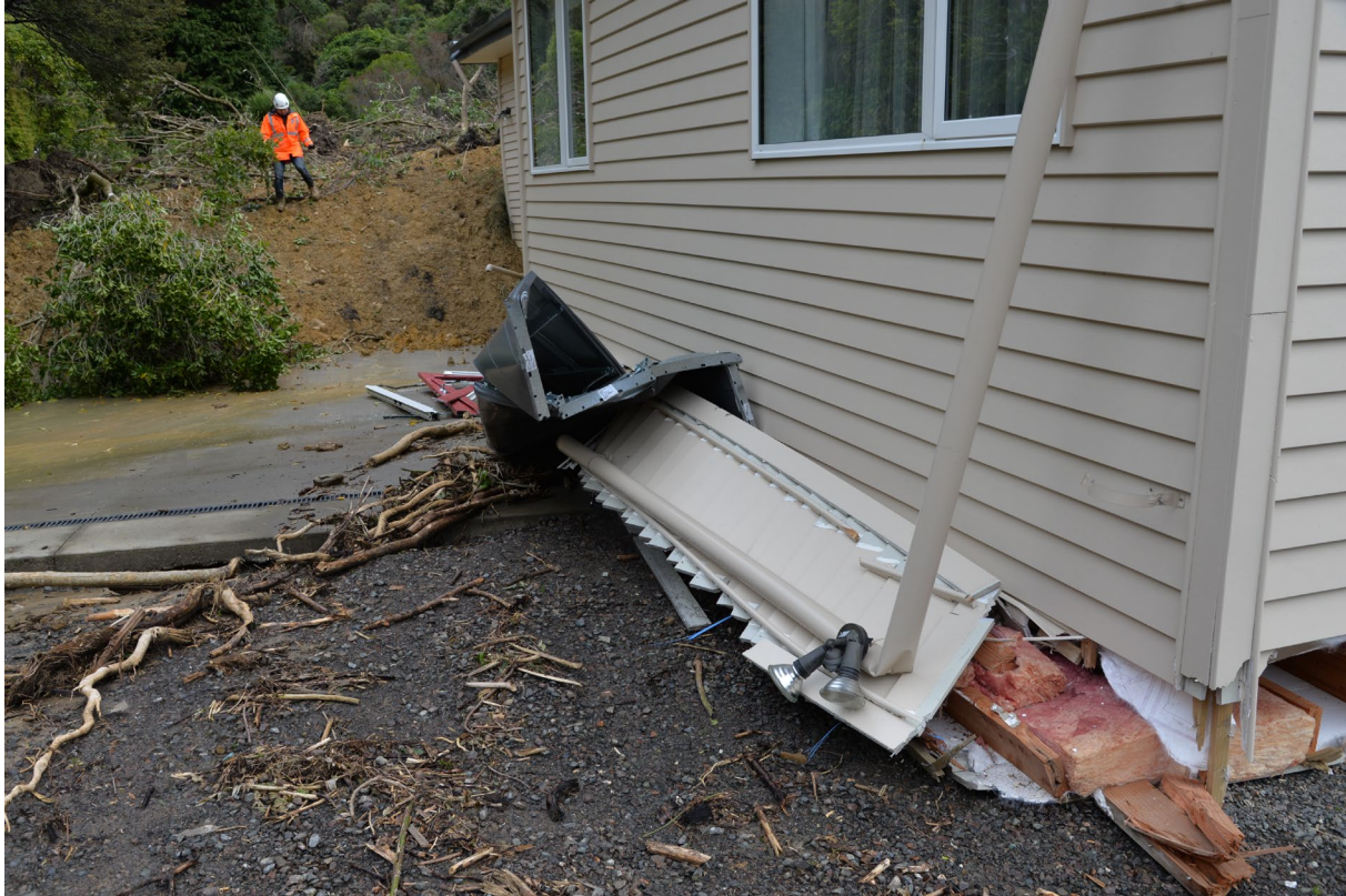
Figure 2.6 Inspecting and assessing structural damage to a home impacted by a debris avalanche.
