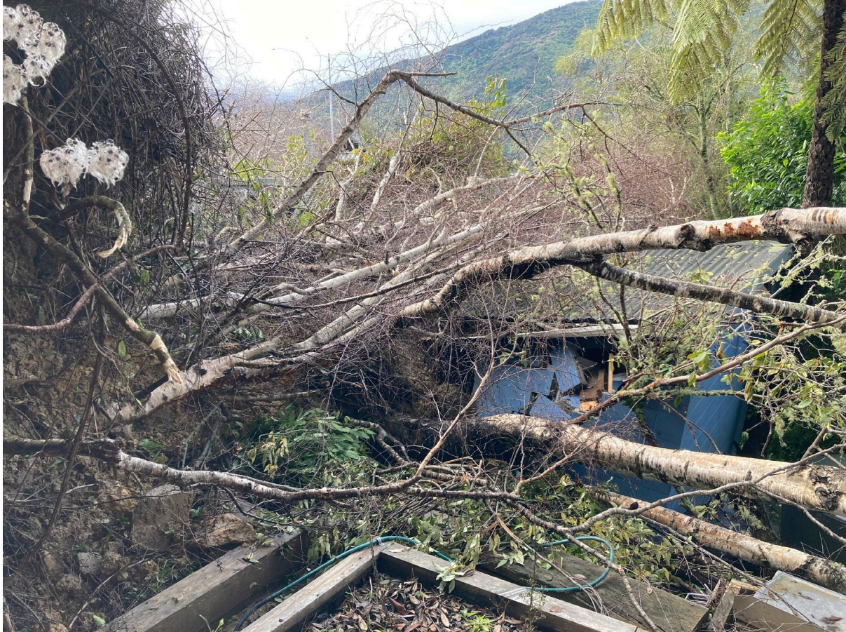
Figure 4.2 Damage to a building from large woody debris.
