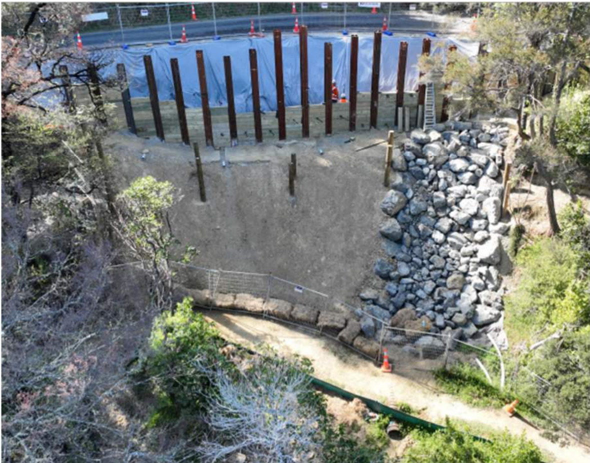
The Aussie Bay site with well installed sediment fence at the bottom of the work site, and secondary protection of hay bales used during concrete pouring and before slope stabilisation is completed.
