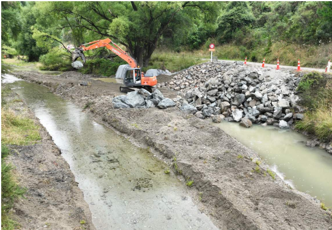
Rock placement occurring on Waikakaho Road with river diversion in place and running clear
