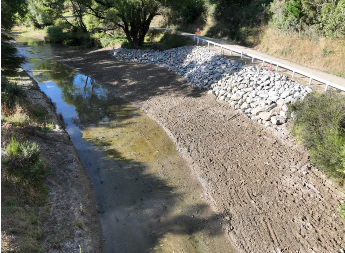
Site completed on Waikakaho Road and river diversion removed and running clear
