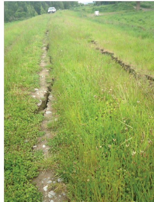
Cracks in the stop bank following the 2016 earthquake and 2021 and 2022 floods
