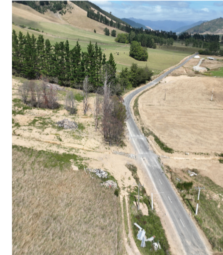
Recovery repair works at the Ronga Road slip site are now complete
