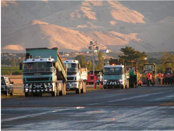
Resealing the Marlborough Airport Limited's runway, Woodbourne (photo courtesy of Fulton Hogan Limited)
