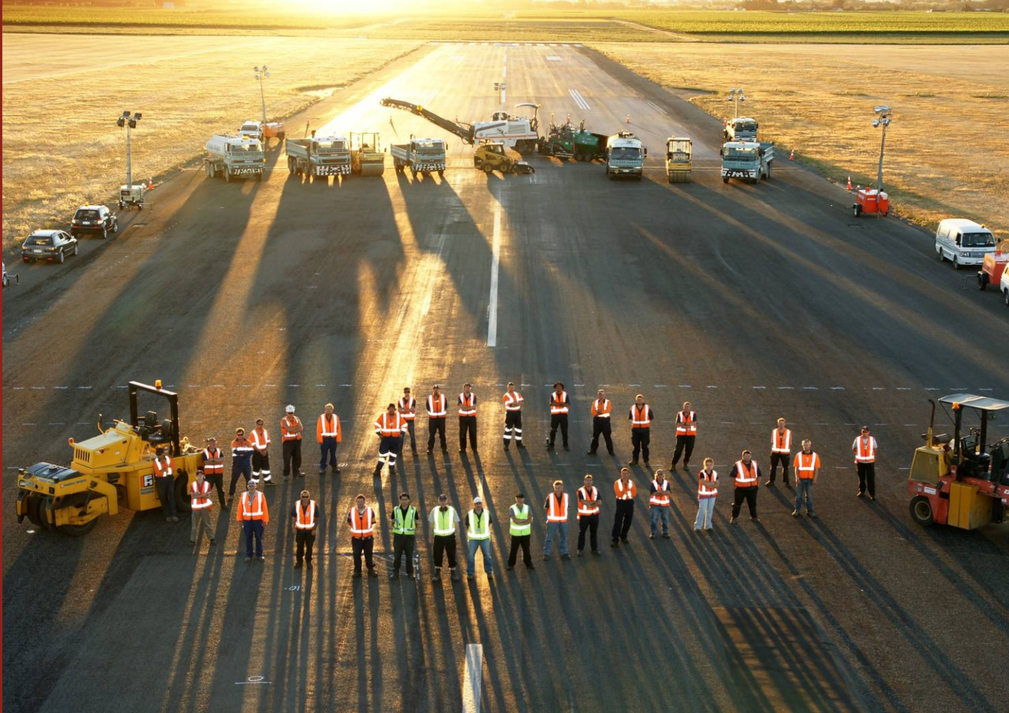
Picture: Resealing Team on the Marlborough Airport Limited runway, Woodbourne (photo courtesy of Fulton Hogan Limited)
