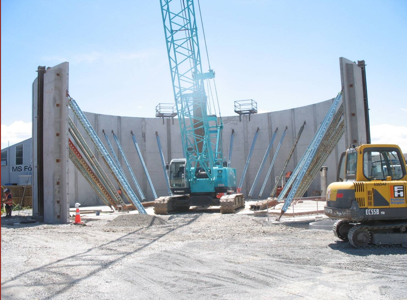
Picture: Construction of the Blenheim Central Water Treatment plant, Auckland Street, Blenheim
