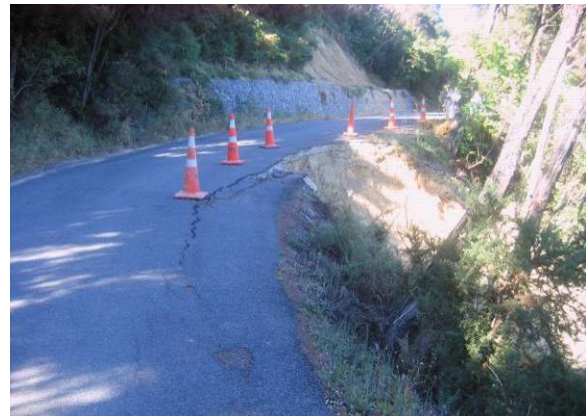
Figure 2: Typical road subsidence damage
