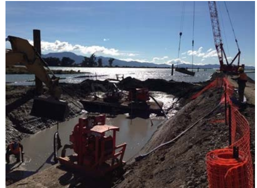
Blenheim Sewerage Treatment Plant major upgrade; the main contractor, HEB Construction Ltd, is shown starting excavation on the landward section of the outfall pipe.
